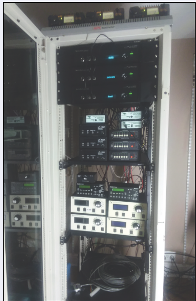
A view of the inside hardware used in the W9SN/4 remote station during the CQWW WPX CW contest.
